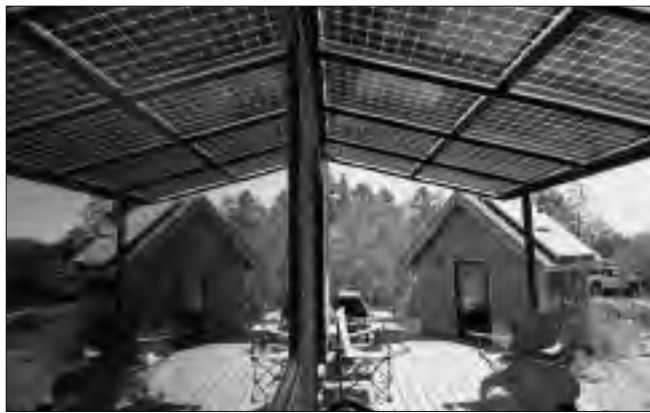
PV Panels serve a dual purpose, generating electricity and providing shade on the porch
