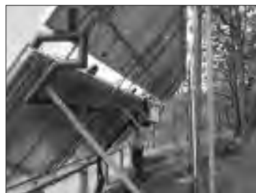
Connecting the panels on an array which illustrates the scale of the project
