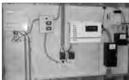
Control Central with the inverters, charge controllers and disconnects
