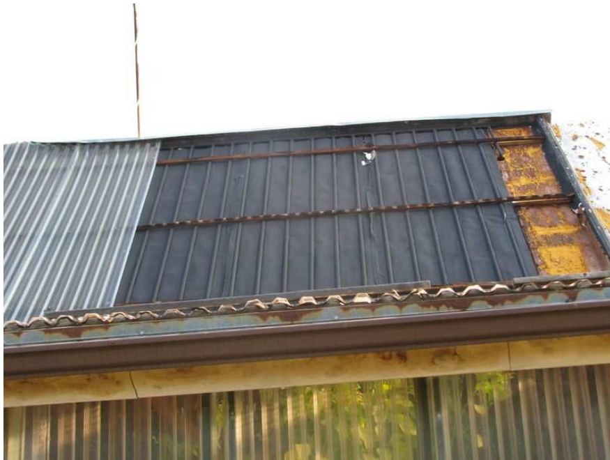
Cover panels removed reveal greenhouse solar hot water collector pipes.
