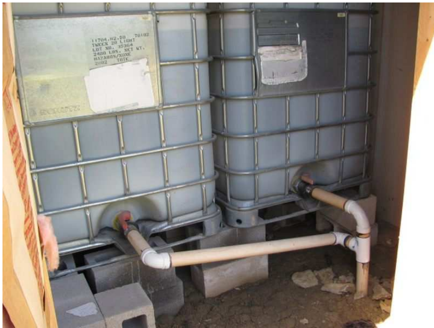
Two 350 gallon tanks plumbed together for increased reserve.
