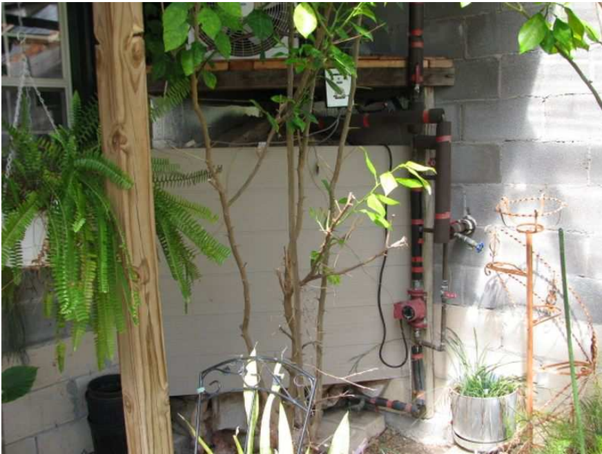
A small pump (red device in line with the pipes) circulates solar-heated water.
