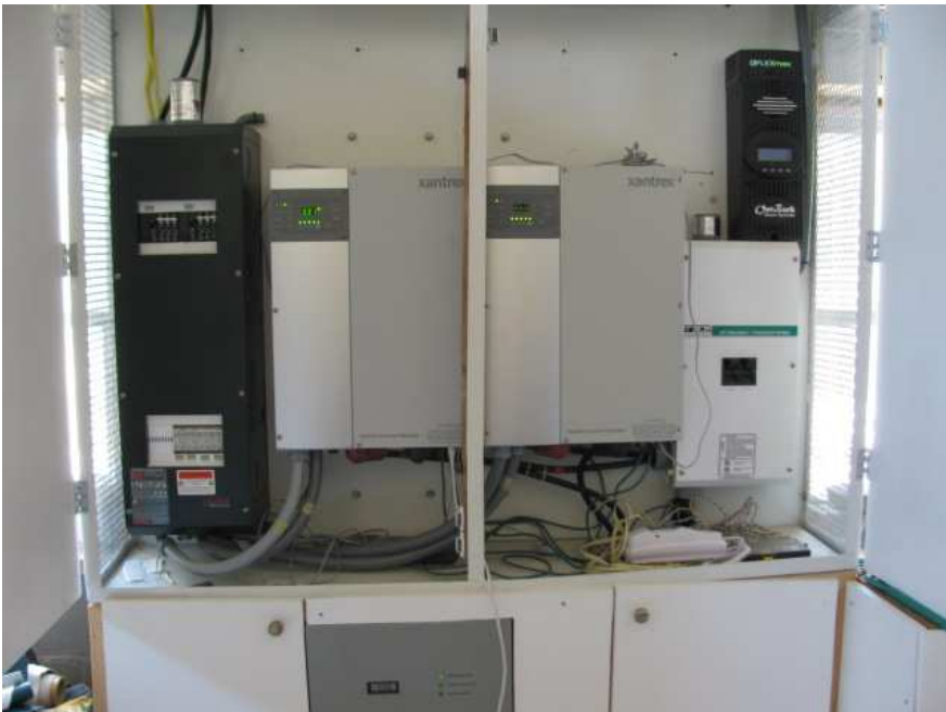
The "business end" of the solar power system inside the custom cabinet.
