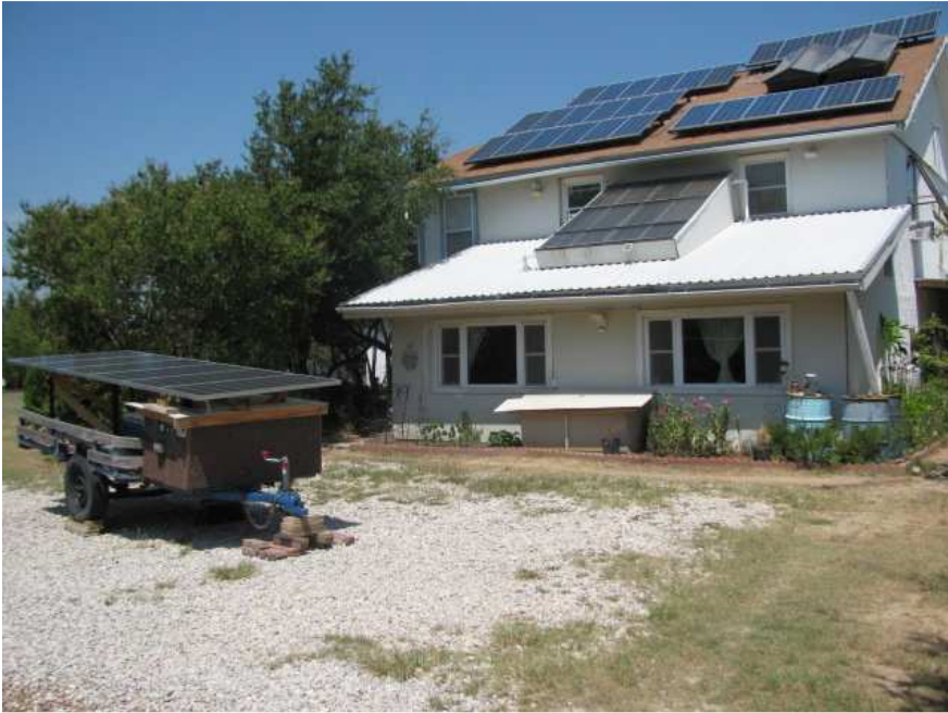
36 PV panels rated 4,520 watts. Average output is 25 kW-h per day.
