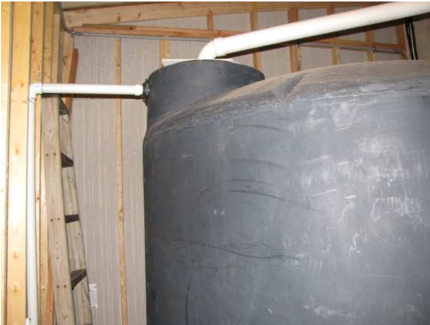
Rainwater enters the top of tank #1....
