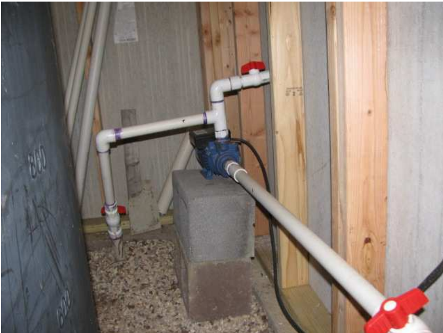
A pump moves the water from tank #2 to where it's needed.
