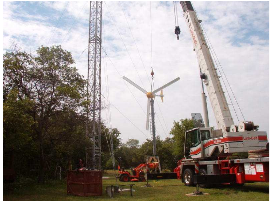
The big lift. A large crane raised the wind generator to the top of the tower.
