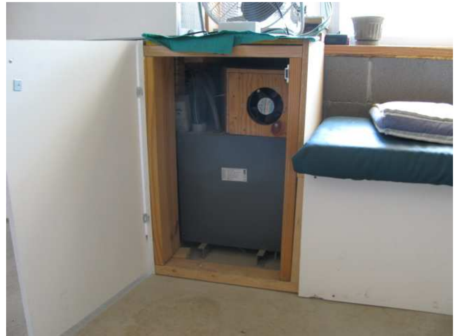
Transformer for wind turbine. (Note the large cooling fan!)
