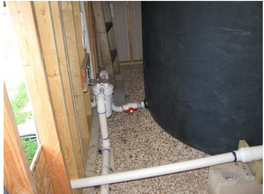
Gravity feeds the water from tank #1, through a filter, and into tank #2.
