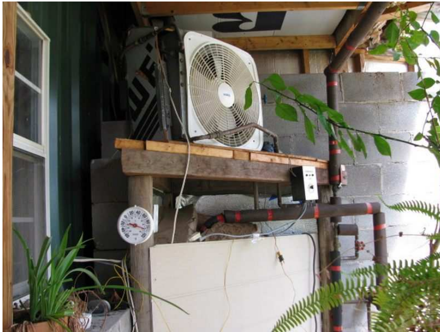
A fan circulates the air in the greenhouse. It's 100°F inside!
