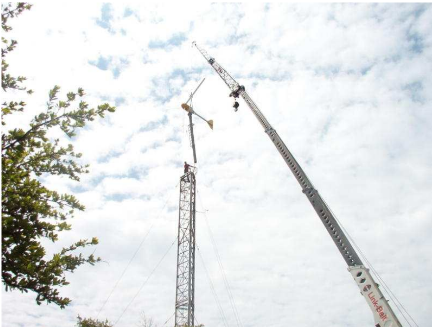
The wind generator almost in place. That's Mike on the top of the tower!
