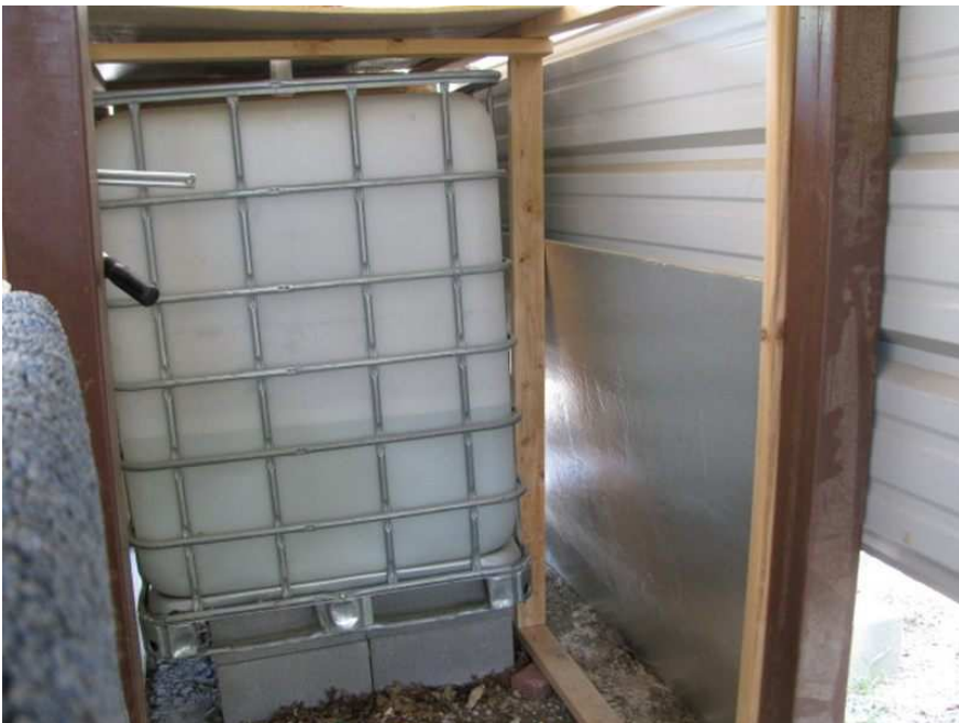
350 gallons of rainwater storage.
