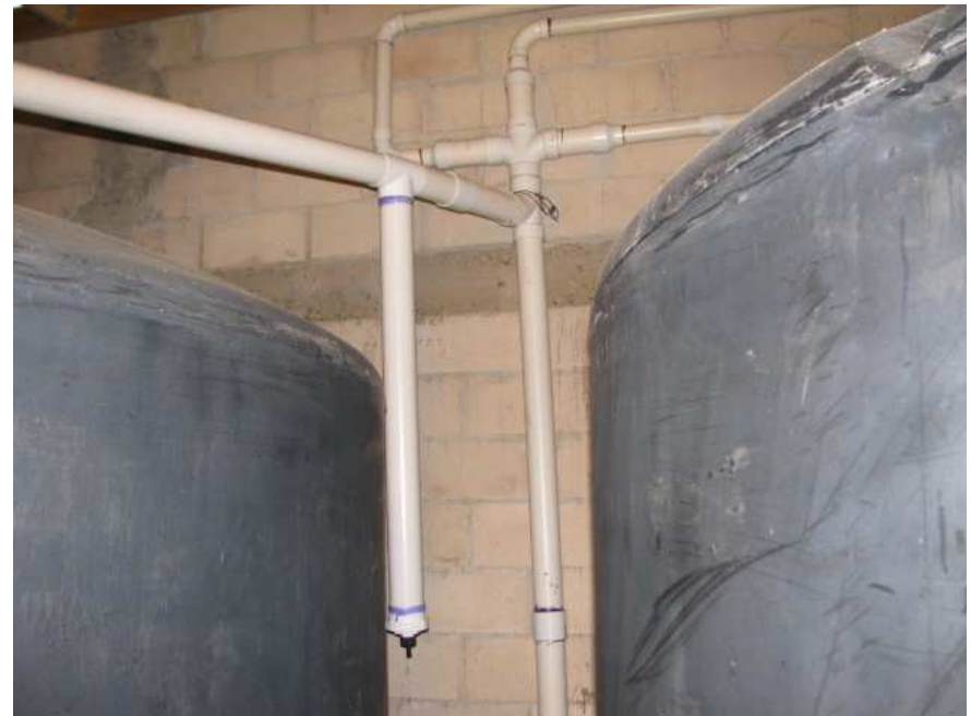
Plumbing routes rainwater from the house roof to dual 2,500 gallon tanks.
