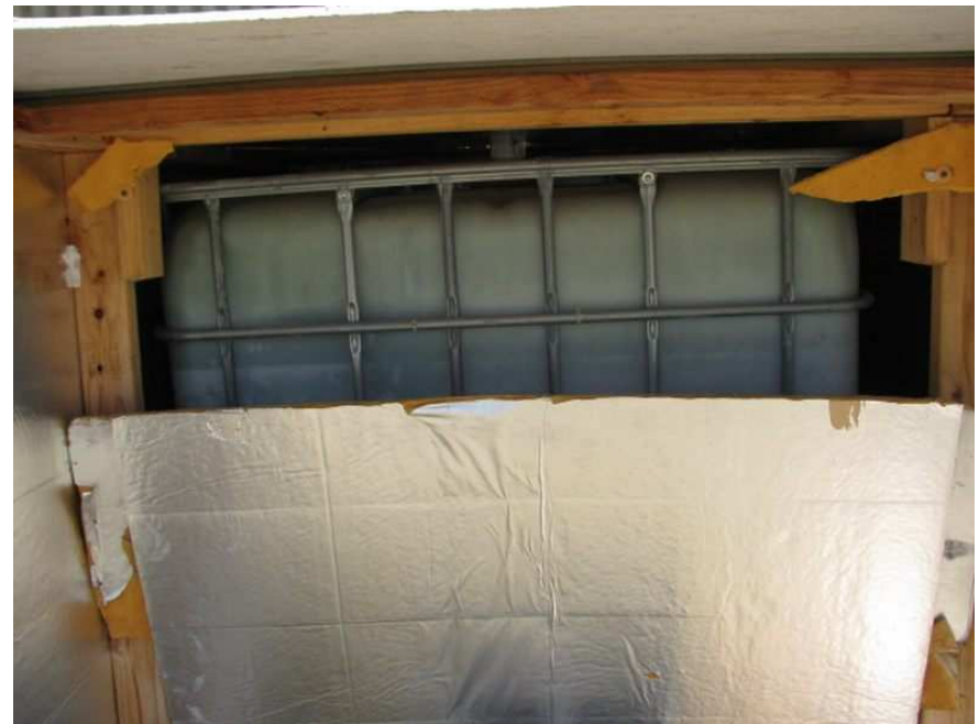
The stored water is insulated to keep it from freezing. It also reduces algae.
