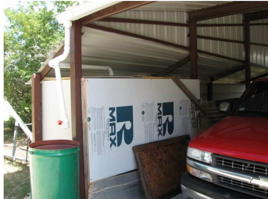
Garage rainwater storage insulated to prevent freezing and algae growth.
