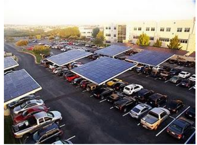
100 kW array at Dell, Round Rock
