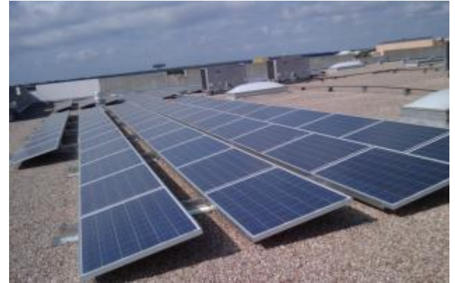
100 kW commercial array, Round Rock
